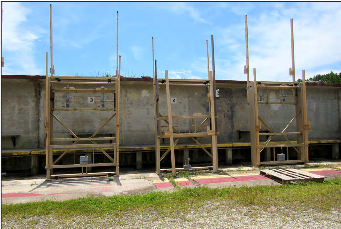
PLATE 21: Range Bravo, Detail of Concrete Wall and Pit with Butts, Looking South, Stone Bay Rifle Range Historic District, Camp Lejeune, North Carolina
