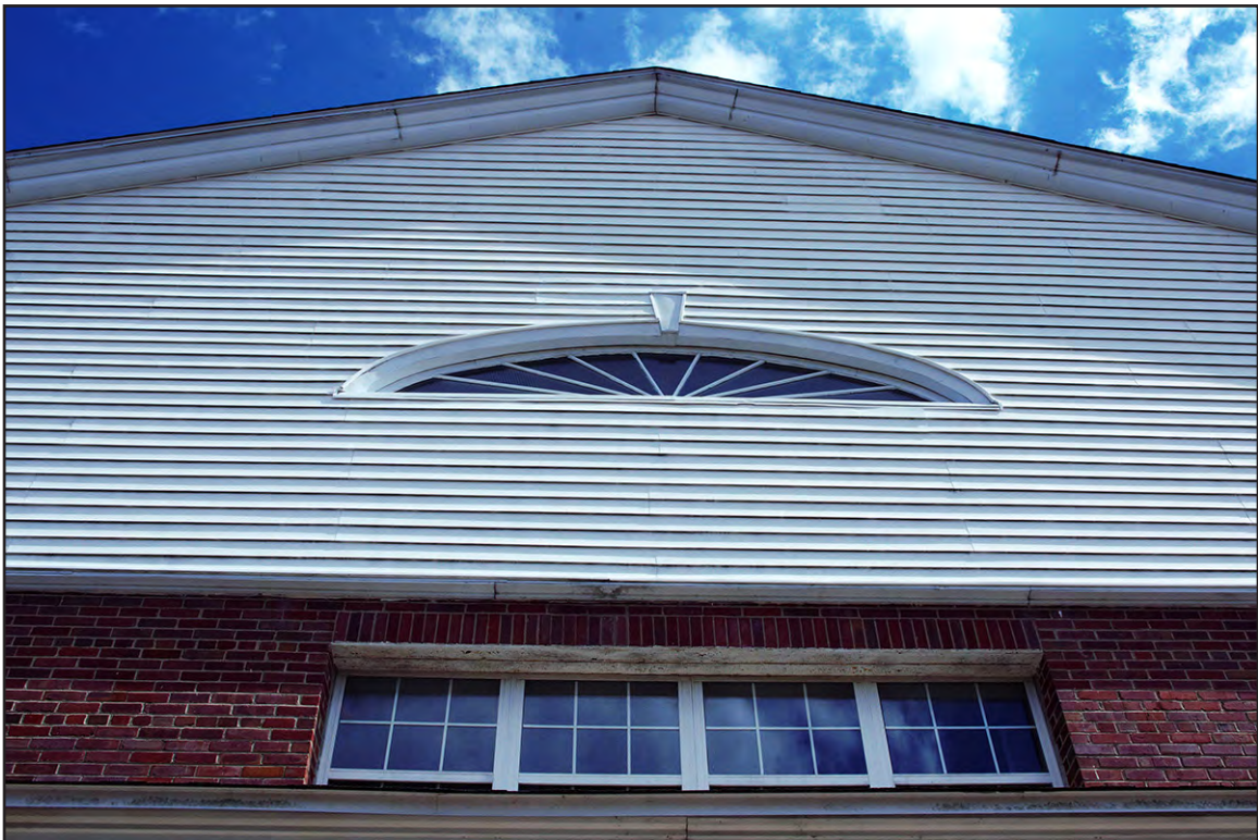
PLATE 17: RR8, Gable End of West Elevation Covered in Vinyl Siding, Typical Treatment of Exterior Wood for Buildings in Stone Bay Rifle Range Historic District, Camp Lejeune, North Carolina
